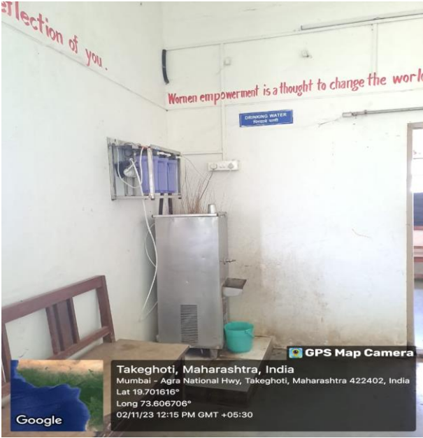
Water Purifier in ladies' common room
